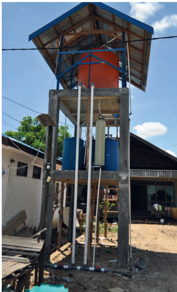
Figure 6: Previous project infrastructure sitting unused (reticulated river water).
