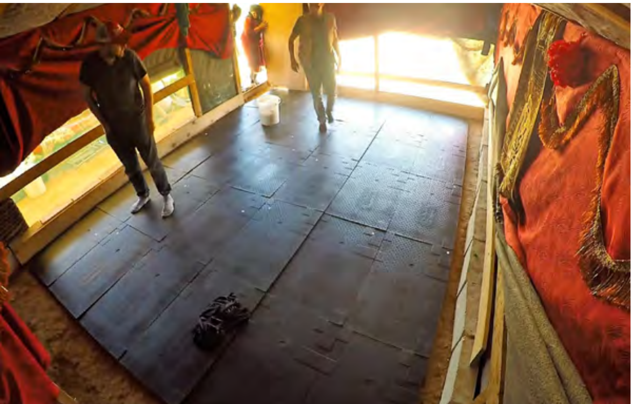
Figure 3 (top): A typical refugee shelter in the selected settlement before Emergency Floor installation
