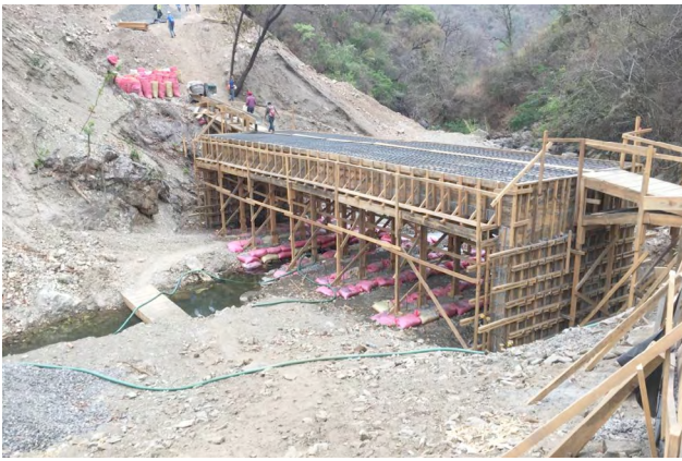
Figure 1: Formwork for the Aguacate II Vehicular Bridge in Joyabaj, Guatemala using locally sourced timber
