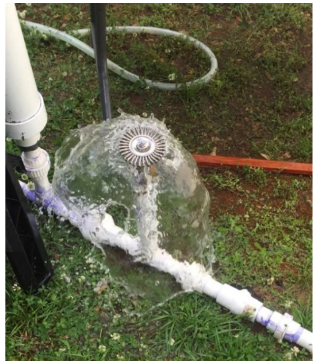
Figure 3: The operating test ram pump
